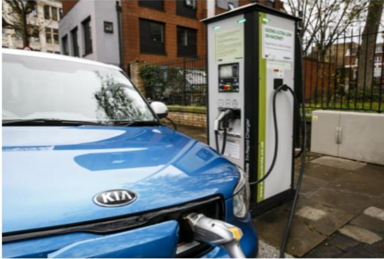
Level -2 Charging (EVSE)
